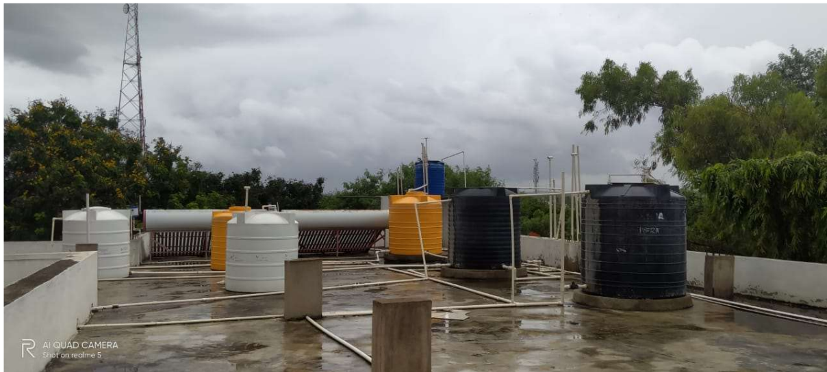
WATER STORAGE TANK ON THE ROOF OF THE HOSTEL FOR DISTRIBUTION OF WATER
