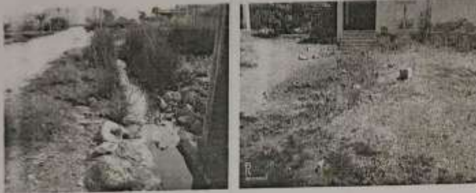
Fig-3 Sewage water flowing at Kandagal road Highway Bi-Pass and in college campus. Time 3:40Pm.
